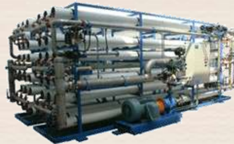
Reverse osmosis unit
